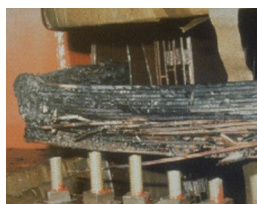
Damaged transformer, Salem nuclear plant, 1989. (Source: Oak Ridge)
